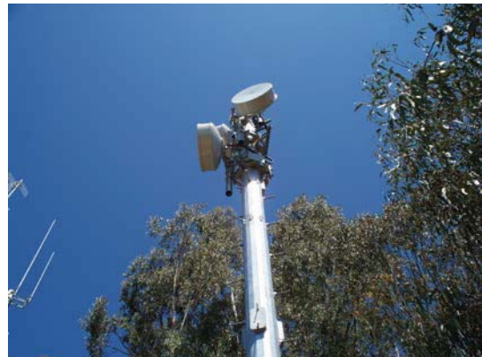
ECOMM Antennae at Eagle Rock
